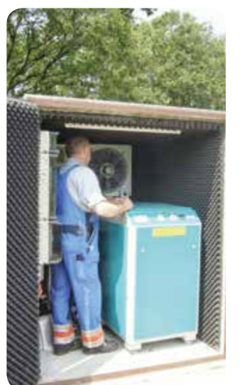
Concrete equipment cabinet
