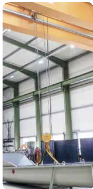
Generous production area with a hook clearance of 8 m
